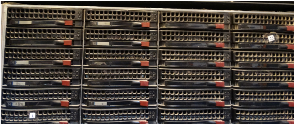
The RAIDIX storage server
